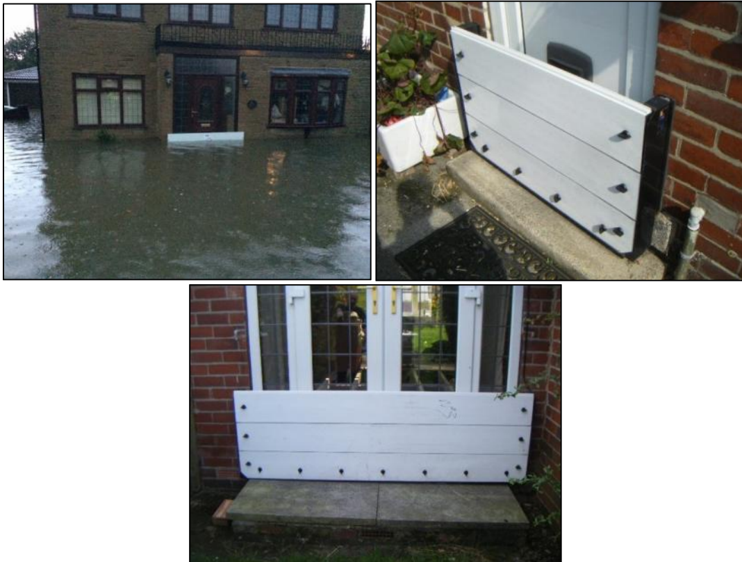
Figure 20: Flood gates in position during flood event and afterwards in West Garforth [reproduced by kind permission of the Garforth Flood Group]
