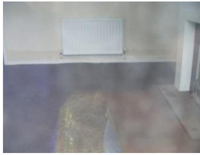
Figure 5: Flood damage to homes in Allerton Bywater. Note tide mark along back wall
