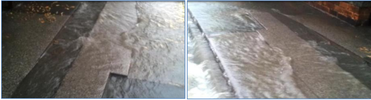
Figure 29: Water escape under pressure along line of culvert
