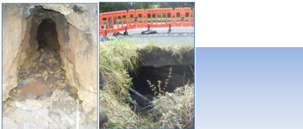
Figure 36: sink hole below B6137, Kippax
