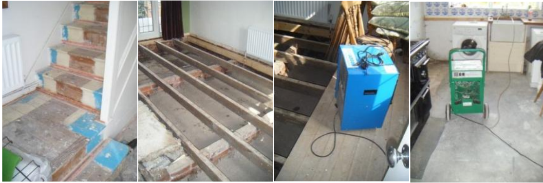
Figure 18: Flood damage to homes in West Garforth
