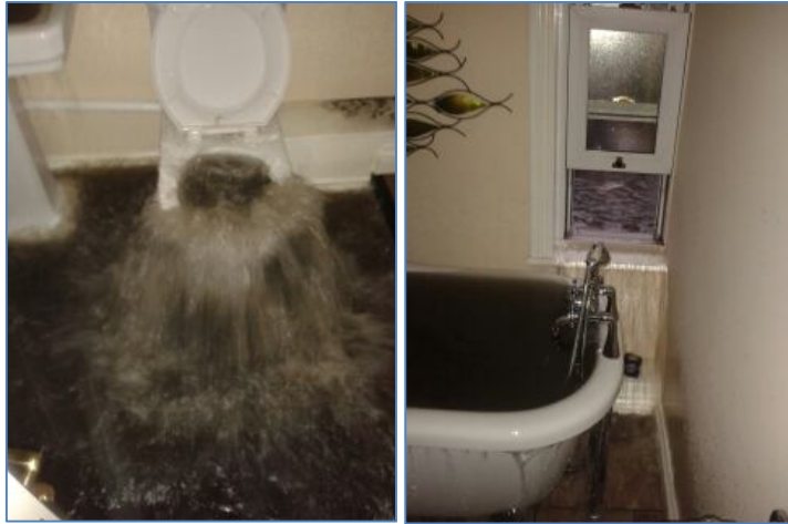
Figure 31: Internal flooding caused by sewer surcharge and overload [reproduced by kind permission of the Garforth Flood Group]
