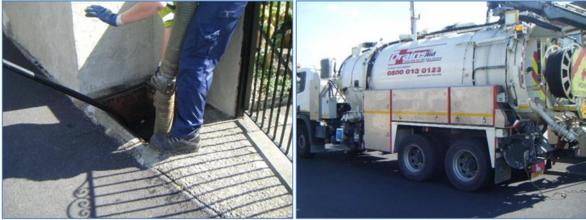
Figure 46: FRM clearing blocked private sewers in The Drive, Saturday 9 th August
